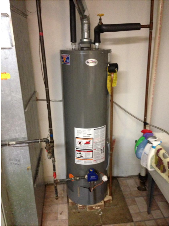
Water Heater Furnace
